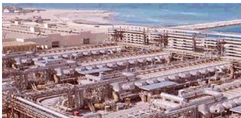
Sea water treatment MSF
